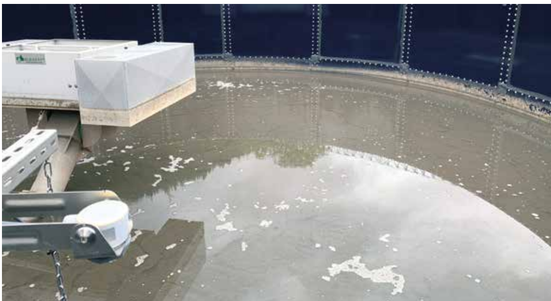
Fig: Application in SoftWater at the SBR reactor in Zernez (SWITZERLAND)
