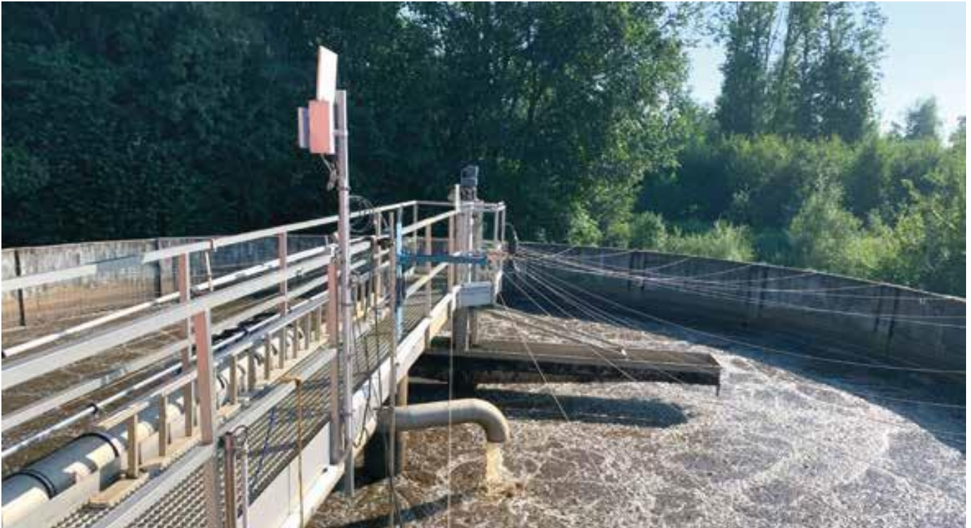
NeoWaterFX300 application in the SBR reactor in Avenches (Switzerland)
